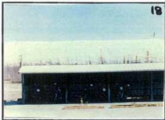
Another horizontal storage tank showing the same signs of condensation and rust as all the others coated with foam.
