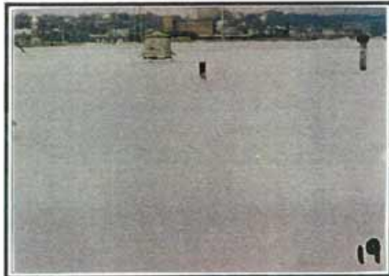
The top of a moving and storage building in Moline, Illinois. The roof had leaking problems and was structurally faulty. SUPER SEAL TAPE (36" width) was applied over the existing tar first, then overcoated with SUPER THERM. This stopped leaking and helped to insulate the building.
