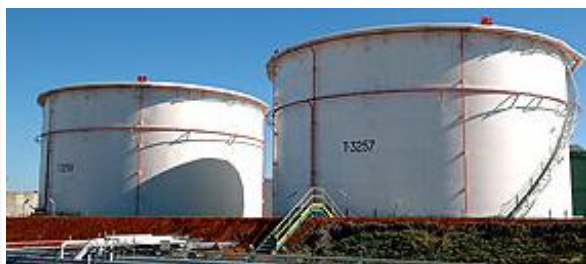
White coated storage tanks
