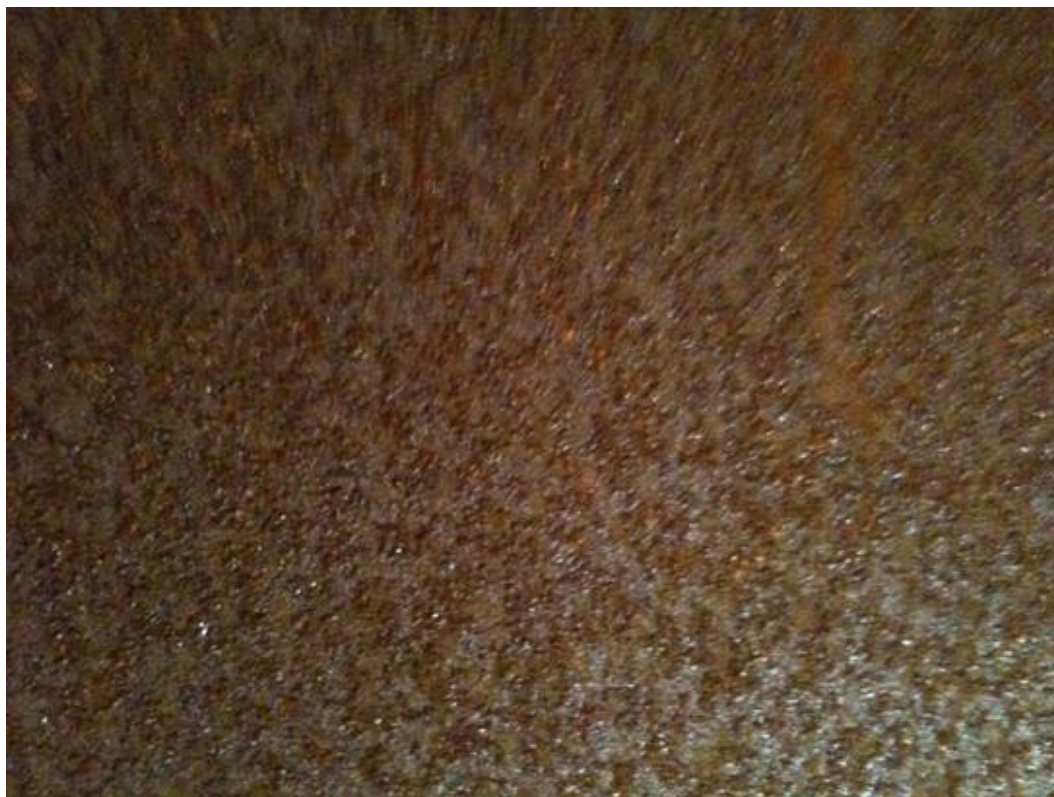
Flake rust corrosion profile on the walls before wire brush.
