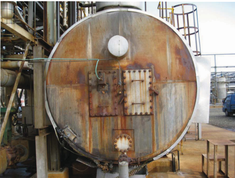
Incinerator Before: 180^{\circ}\text{C}
