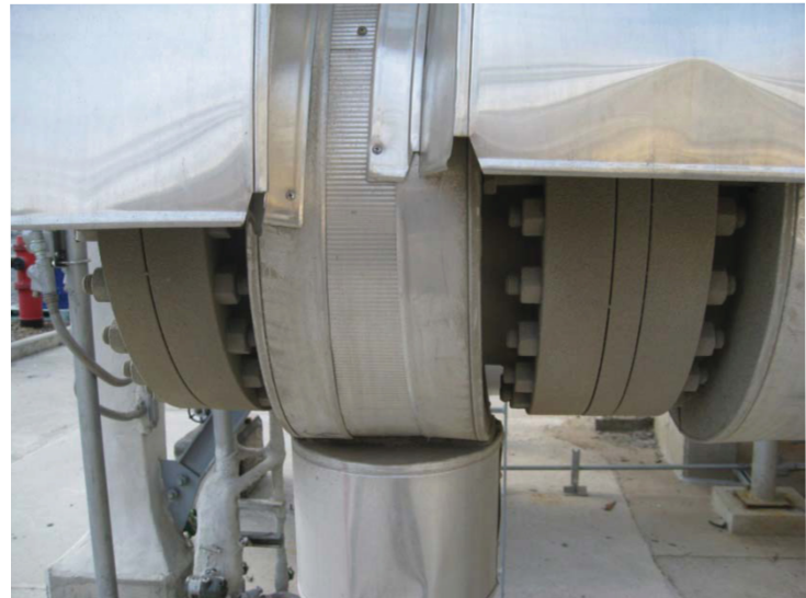
Flange After coating: 45^{\circ}\text{C}
