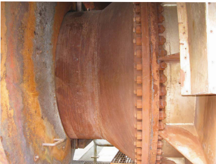
Incinerator Before: 260^{\circ}\text{C}
