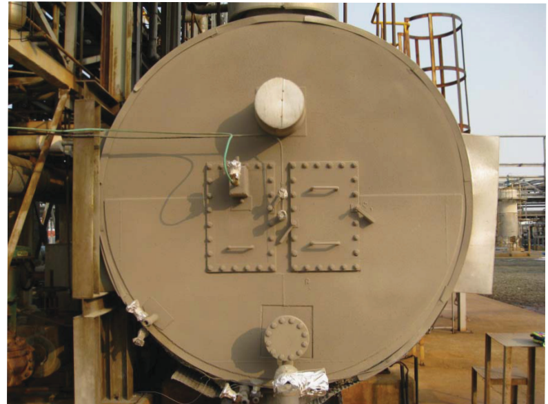
Incinerator After: 50^{\circ}\text{C}
